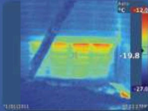
Thermal Image shows heat loss due to lack of insulation
